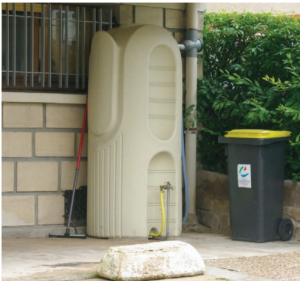
Figure 2. A rainwater harvesting tank installed by the DSEA.
