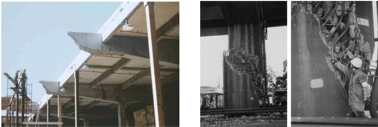
Figure 2-34: Partial collapse of reinforced concrete structures by shear failure, Air Force warehouse 1955 (USA) on left, a bridge pile after the seism in 1995 at Kobe (JPN) on right.
